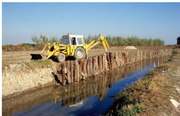
Wall made with natural material for the protection of the slope in the outer channel of the wetland (Author: CCEDCV)
